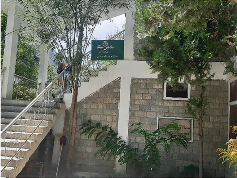
Image 8.3 A Family Planning Center in Gilgit Baltistan, the staircase of which can be a barrier to access
