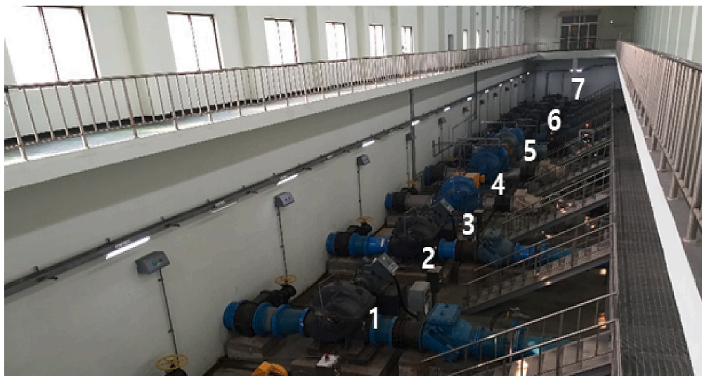
Fig. 2. The water supply pump station used as test bed.
